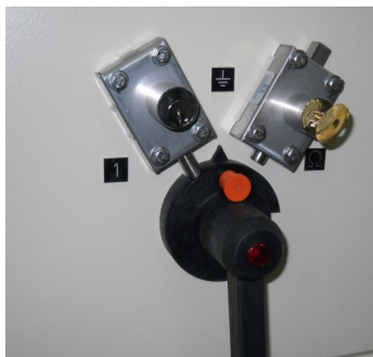
Isolating and earthing switches with lock
