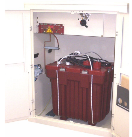
PTS32 ext XL with 16 kVA transformer
