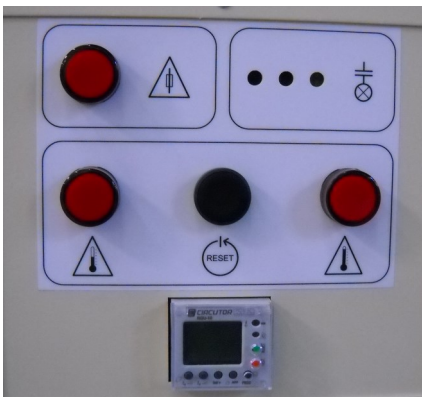
Signalling and control panel
