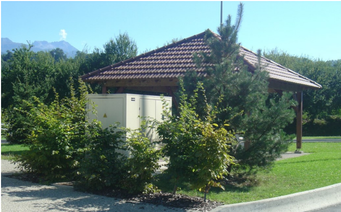
Aire de la Clusaz, supply to rest area
