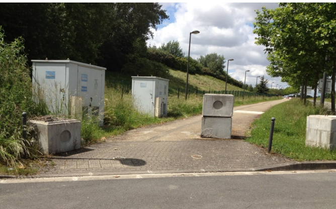
Carole race track, lighting supply
