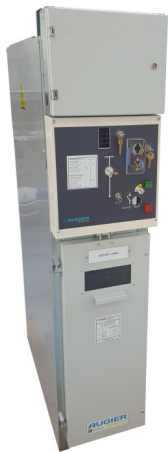
Picture : On load switch panel
