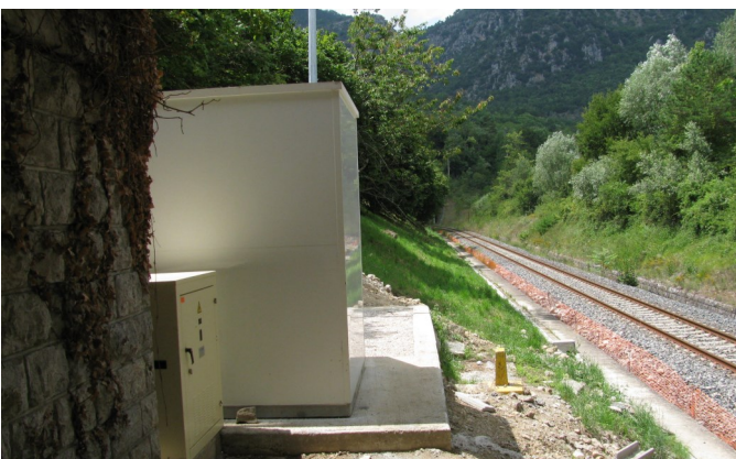
Tunnel de Braus, communication GSM-R
