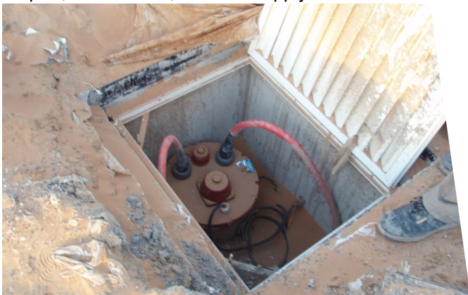
Airport, Middle East, lighting supply
