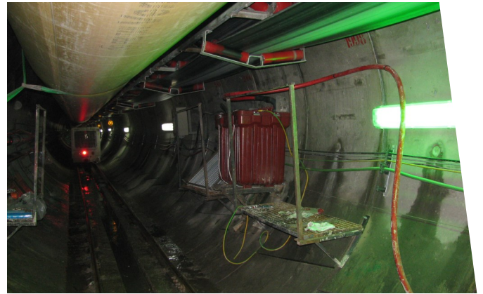
Tunnel, Spain, lighting and outlet supply
