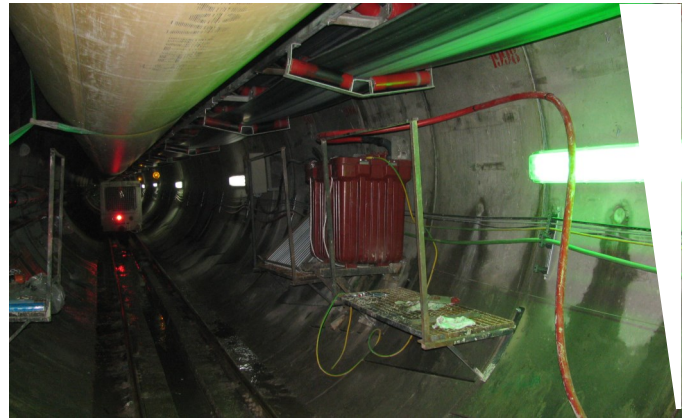
Tunnel, Spain, lighting and outlet supply
