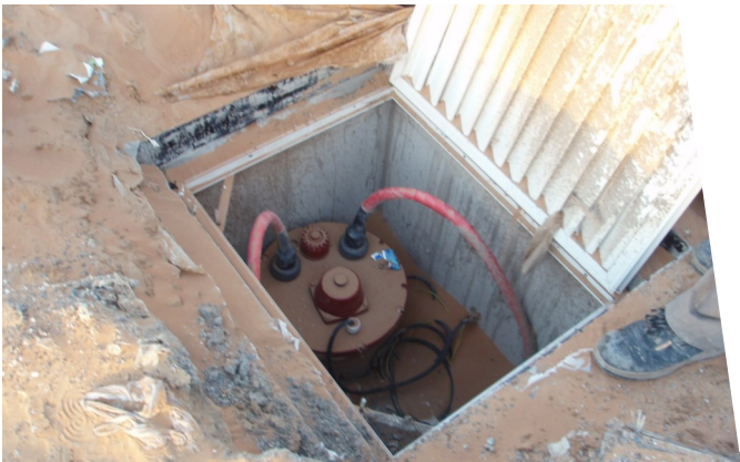
Airport, Middle East, lighting supply
