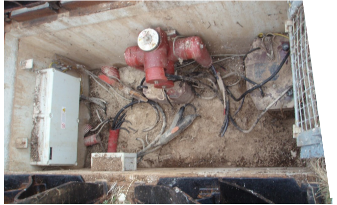
Large sites, France, car park lighting
