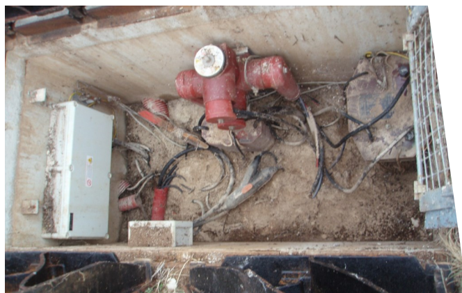
Grands sites, France, éclairage parkings
