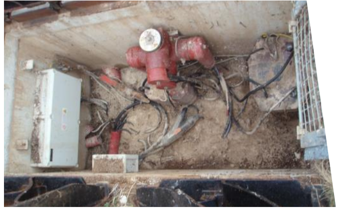
Large sites, France, car park lighting
