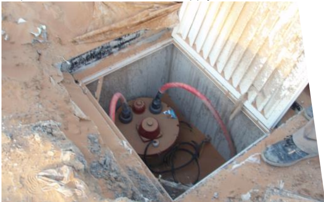
Airport, Middle East, lighting supply
