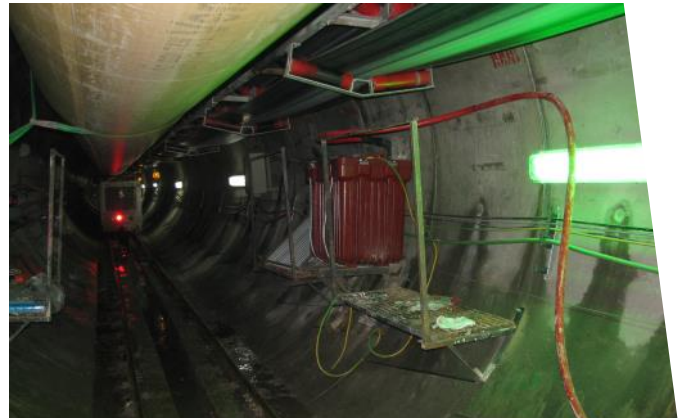
Tunnel, Spain, lighting and outlet supply
